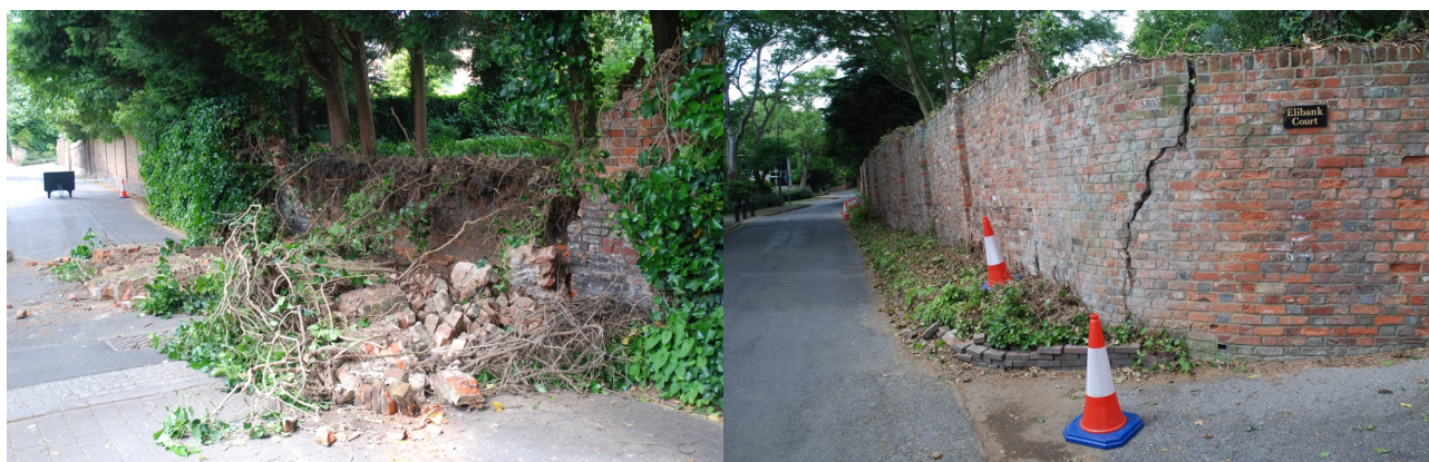
Elibank Court's Cracked Wall
